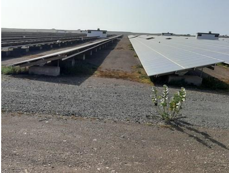
Figure 2- 2- Example of photovoltaic panels and respective support structure; transformer cabins in the background (Sal island)
