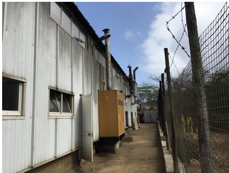
Figure 3- 6- Generating set exhaust chimneys at Favatal Power Station
