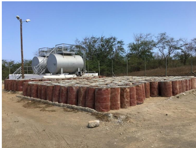
Figure 3- 5- Fuel storage at the Favatal Power Station
