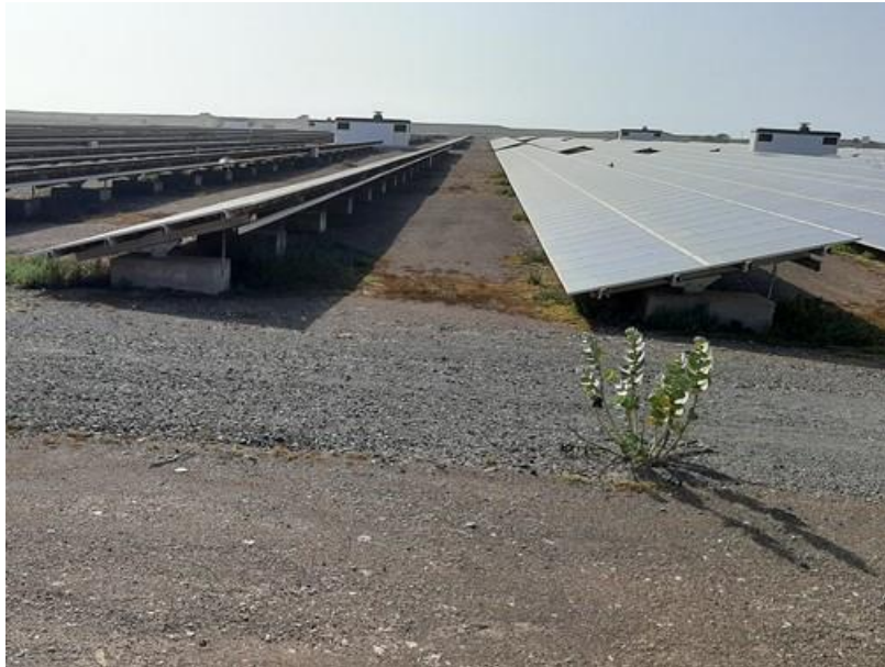
Photo 1 - Solar PV panels and support structure set in concrete blocks (Sal Island)
